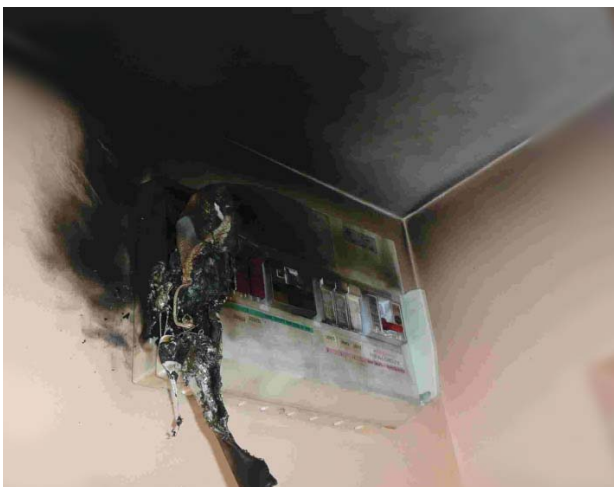
Result of a DIY home owner having wired an 10.5 kW electric shower circuit with 2.5 mm 2 cable and a 45 A circuit-breaker. (Photo courtesy of British Gas)
